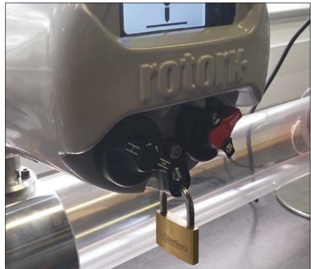
Fig 7.2. IQ3 control selector padlocked in "Remote"
