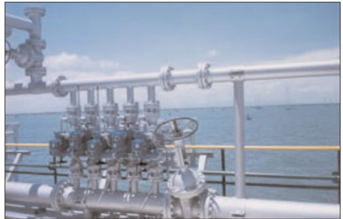
One of the many flow station valve manifolds on Lake Maracaibo that have been automated with Rotork Q range actuators and Pakscan two-wire control.
