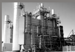
Rotork actuators are used by Colorado Energy Management.
