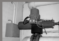
Rotork Skilmatic self contained electro-hydraulic actuators in use at Wyoming water treatment plant.
