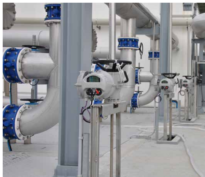
IQ actuators installed at Viseu Sul WWTP.
