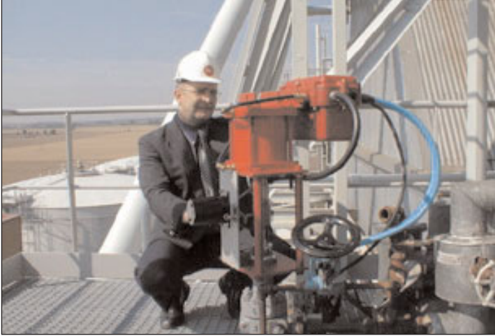
Sales manager Ian Elliott attends to the commissioning of a Rotork Skilmatic SL411 linear actuator on a modulating control failsafe application at Brigg Power Station.
