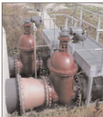
Rotork IQ35 actuators with Profibus connectivity at Ketelmeer.
