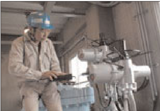
Senior sales engineer Fumihiko Nishimura completes the commissioning of IQ20 actuators at Hachinohe.
