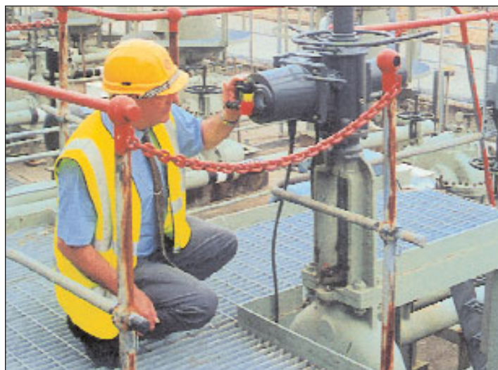
Above: Mike Ling, manager for Shell at Gatwick, with a Rotork IQ25 installed in the tank farm area.
