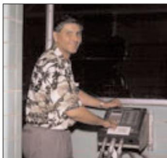
David Milcinovic uses a Pakscan 2S unit to control Rotork actuators in the filtration building
