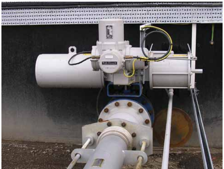
At this refinery in Scotland gate valves have been replaced by triple-offset butterfly valves with Skilmatic EH failsafe electro-hydraulic actuators for ROSoV duty.
