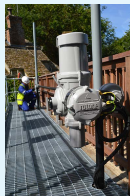
Installation nearing completion on the new walkway platform; the IQ3 actuator in the foreground is fitted with its vandal-proof cover.
