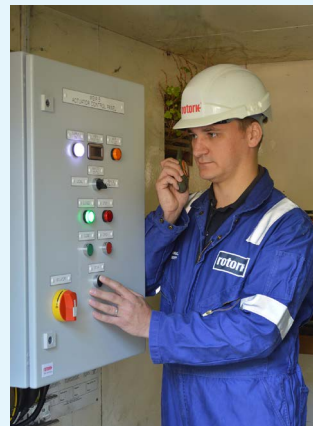
A Rotork engineer confirms the successful operation of the new control panel during site commissioning.
