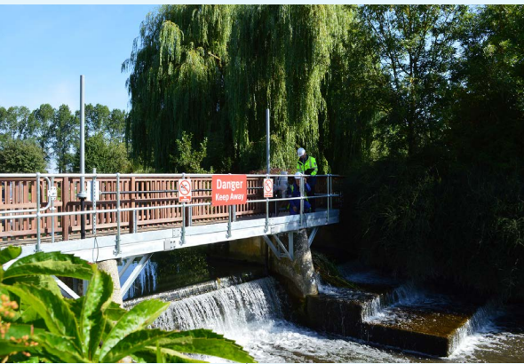
Buscot Weir after the completion of Rotork's extended scope contract, which encompassed project management, new valve actuation and adaptation, a new control panel in an adjacent building and the installation of a new walkway platform for inspection and maintenance.
