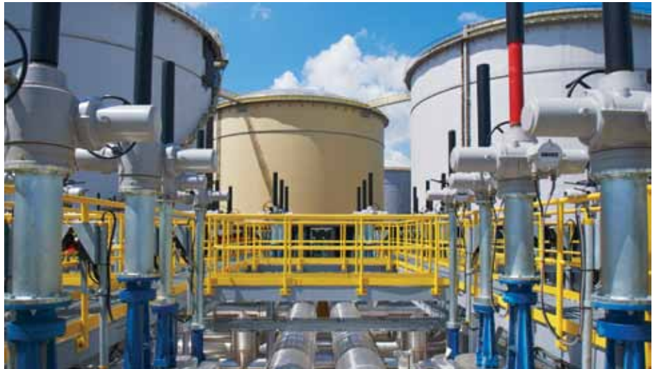
Fig 1: General view of the Vopak Phase 8 plant.
