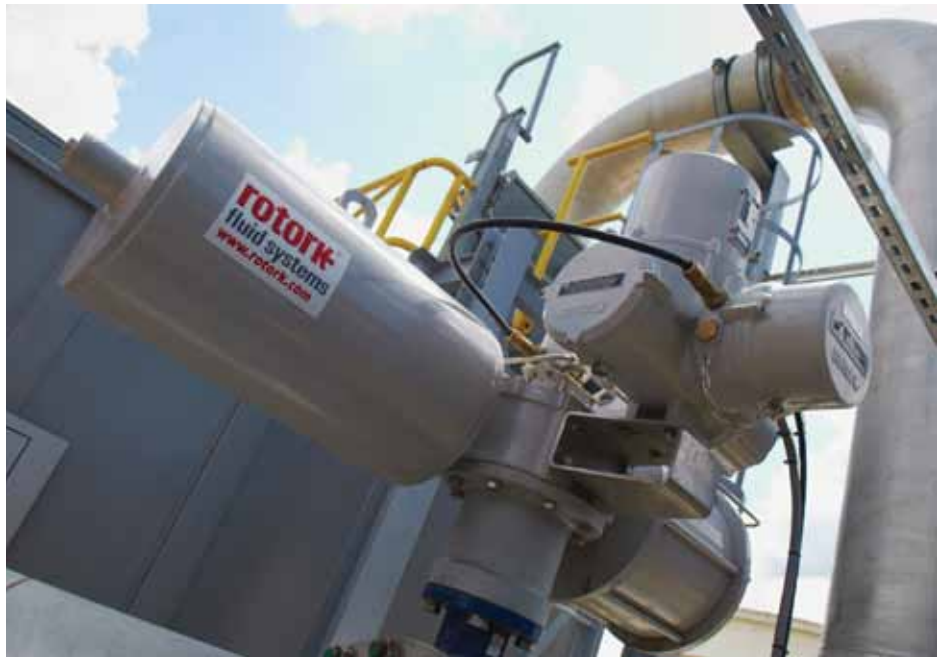
Fig 4: Skilmatic actuator on safety related failsafe valve duty.
