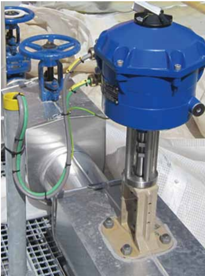
Fig 5: One of the CVL control valve actuator installations at Vopak Phase 8.
