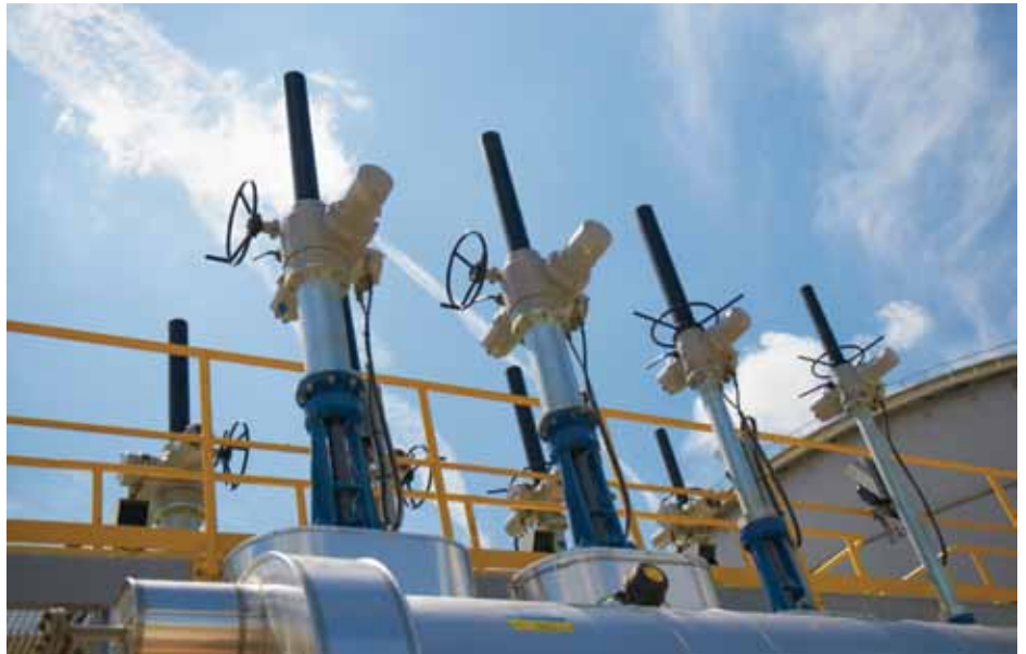
Fig 2: IQPro actuated gate valves on the pump pit manifolds.
