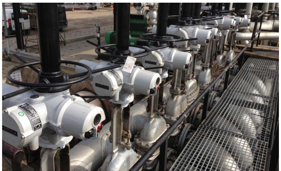
Fig 1: Retrofitted valve actuator installations at the Tupsras Izmit Refinery.
