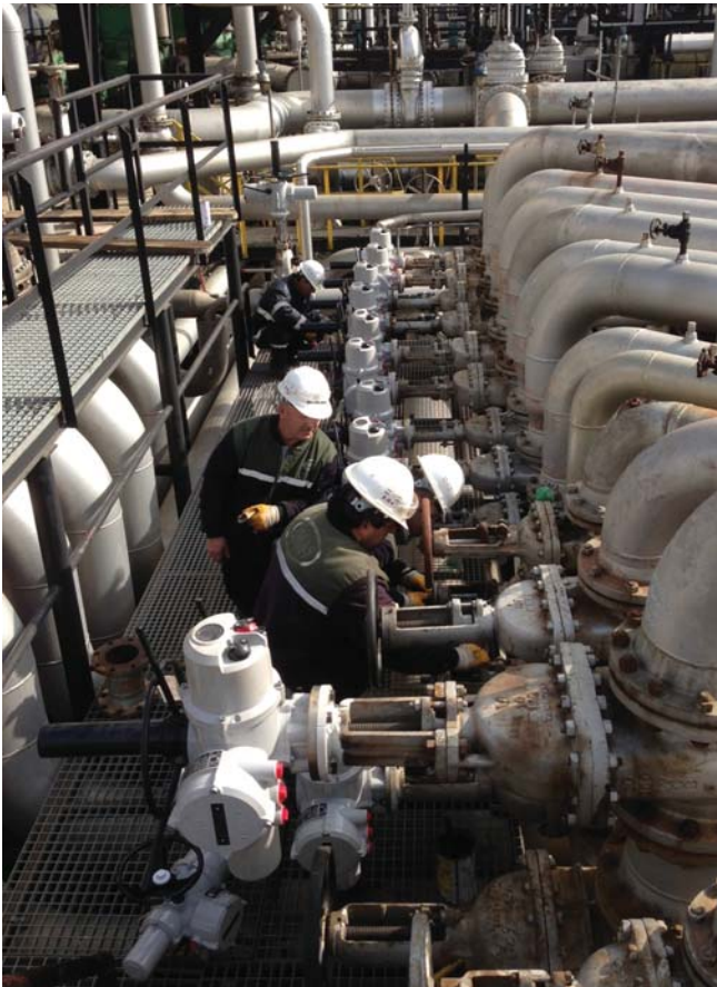
Fig 4: Retrofit work in progress. Engineers from Omas work on one of the tank farm manifolds at the Tupras Izmit refinery. The tank farm upgrade is part of a massive modernisation and expansion programme at the Tupras refinery. This also includes the construction of new refinery facilities on an adjacent site by the Spanish company Técnicas Reunidas, for which more than 400 IQ electric actuators are being supplied through Rotork's Spanish subsidiary company.
