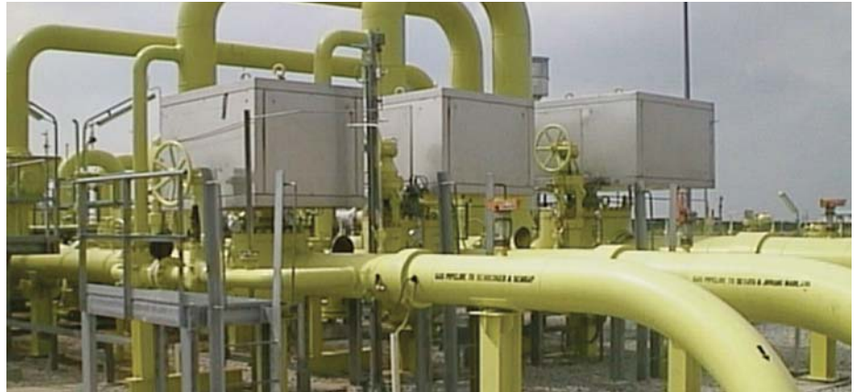
Actuators protected by rigid fireproof enclosures.
