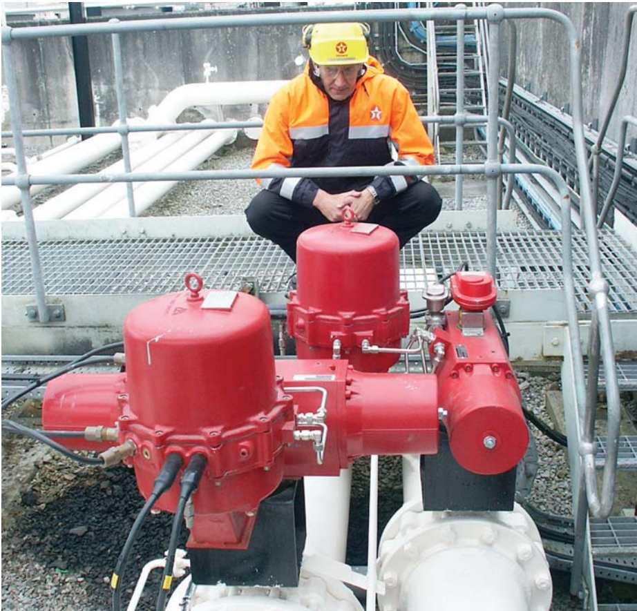
Skilmatic actuators installed at Chevron Texaco, Plymouth, UK.
