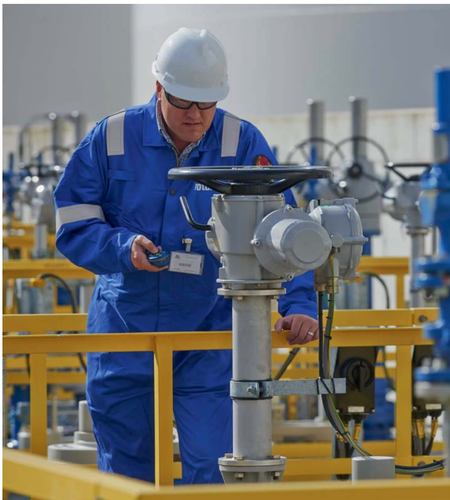
Gathering the data for the Client Support Programme involves a visit to the site, but options to further enhance the service include a direct link between the master station and Rotork via the internet or the cloud.
