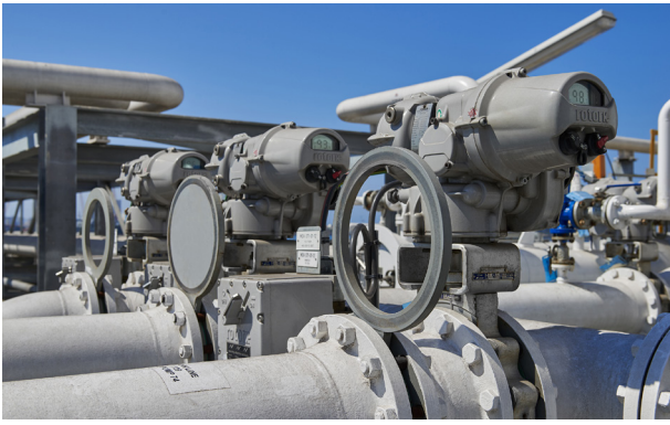
Figure 2. IQT3 Shutdown Battery actuators at a tank farm.
