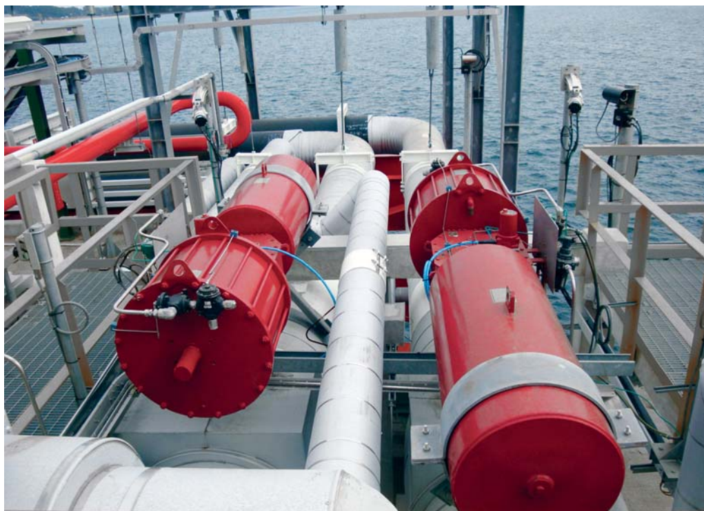
Heavy-duty scotch yoke actuators operating cryogenic service ball and butterfly valves at a marine terminal.
