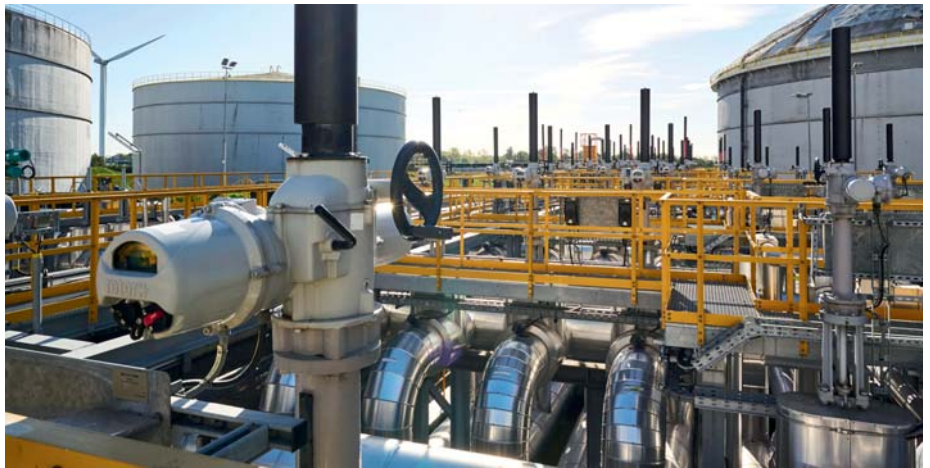
Intelligent actuators on site at a terminal
