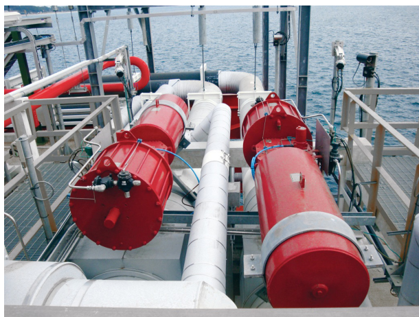
Figure 2. Scotch yoke actuators in service at a marine terminal.
