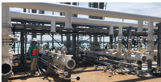
Figure 1. Intelligent actuators in operation at a terminal.
