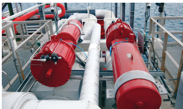
Figure 2. Scotch yoke actuators in service at a marine terminal.
